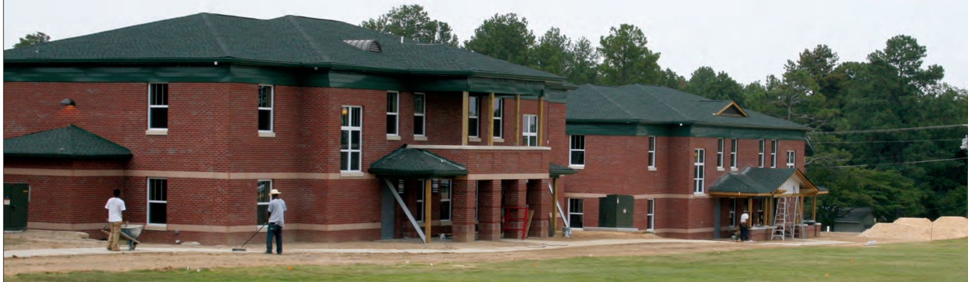
Workers put the finishing touches on two of the new village houses. A total of four village houses were built this summer next to Coach Sink Field, adding 100 beds for on-campus residency.
