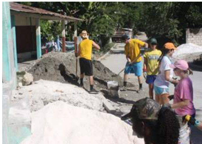
Left, Peter Wildeboer, Josh Clarke, Katie Nation, and Nicole Hardin help build a church office in Haiti.
