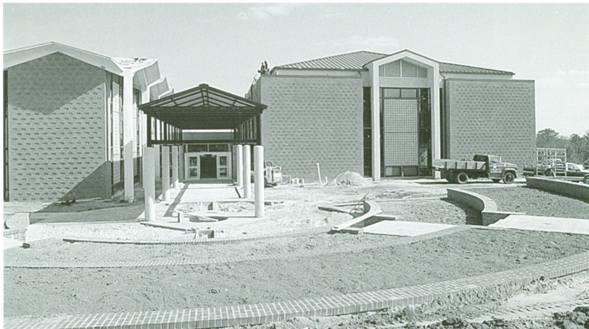
Construction on the annex to Davis Memorial Library nears completion. The plaza entrance will contain engraved bricks honoring alumni, faculty, and many friends of the college.
