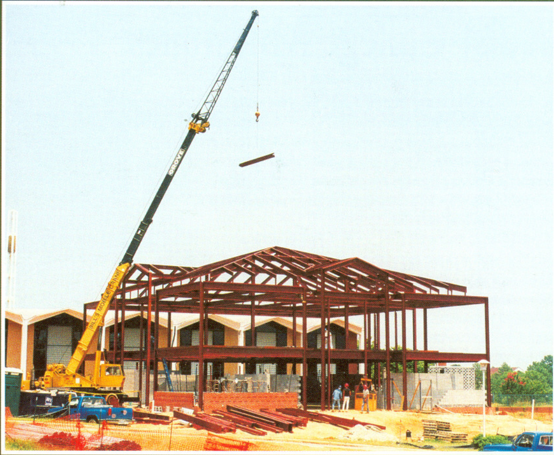
Workers install the steel framework for the annex to Davis Memorial Library.
