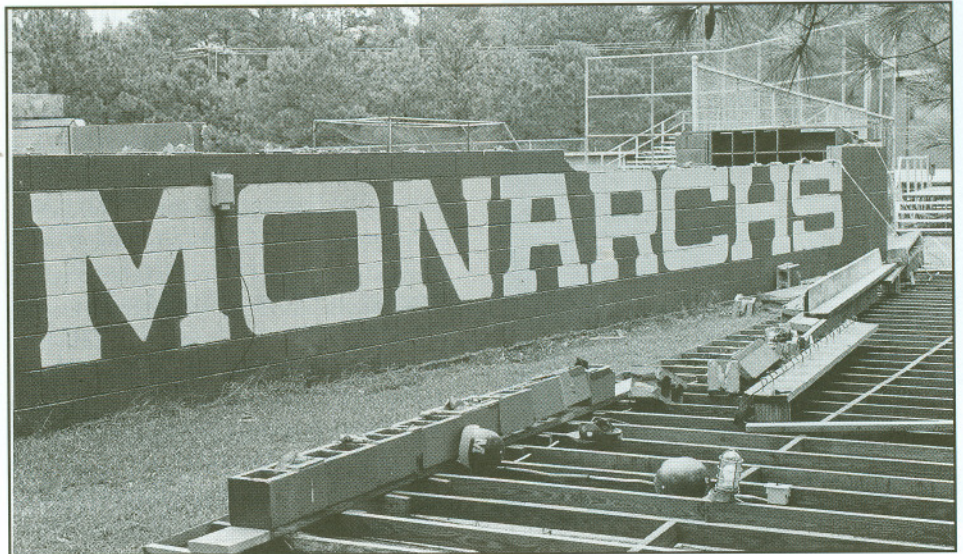
The hurricane lifted the roofs off the baseball and softball dugouts and blew down scores of trees across the campus.
