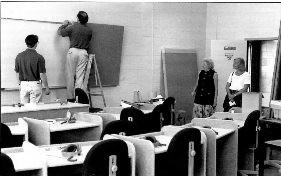
Mrs. Elaine Porter and Dr. Joan Bitterman watch as a workman installs a bulletin board in the newly renovated Language Lab.
