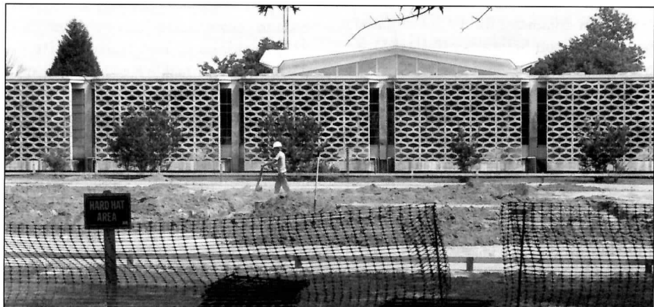
The foundation for the new Math and Computer Science Building is now being laid.
