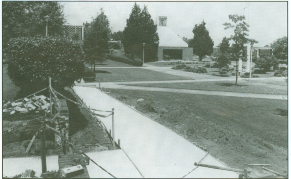
A NEW RAMP ALLOWS MOVEMENT FROM THE FOUNTAIN LEVEL OF THE CENTRAL MALL TO THE LIBRARY LEVEL WITHOUT USING STEPS.
