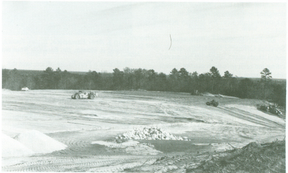
EARTH MOVERS SWARM OVER FIELDS 7 AND 8. THE COLLEGE GOLF COURSE IS LOCATED IN THE VALLEY BEHIND THE TREES. THE PHOTOGRAPHER WAS FACING EAST, NORTHEAST.
