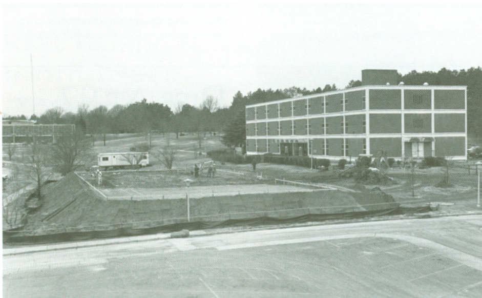
WORKMEN STAKE OUT FOOTINGS FOR THE NEW RESIDENCE HALL. THE CONTRACTOR WAS GREETED WITH SNOW THE FIRST DAY ON THE JOB—DECEMBER 23. BUT THE BULLDOZER PROCEEDED.
