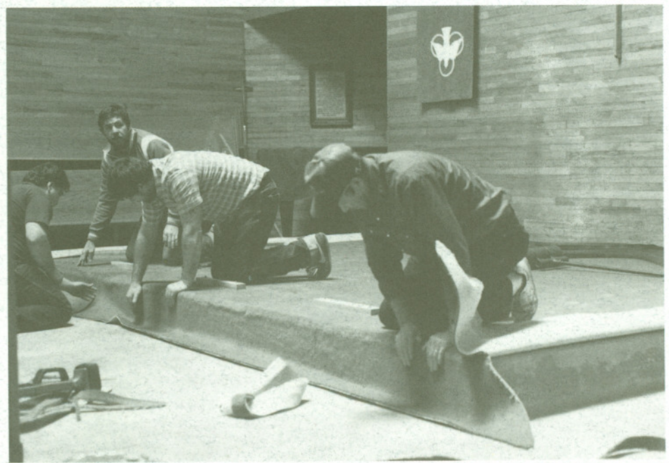
Workers install new carpet in Hensdale Chapel, a gift made possible by Ruth Palmer of Kitty Hawk, N.C.
