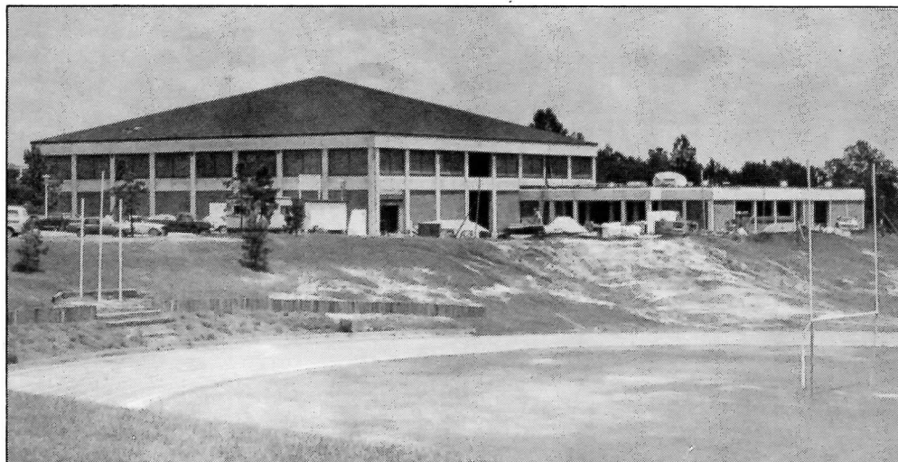
Below - Construction of the Physical Activities Center is on schedule for completion in December.
