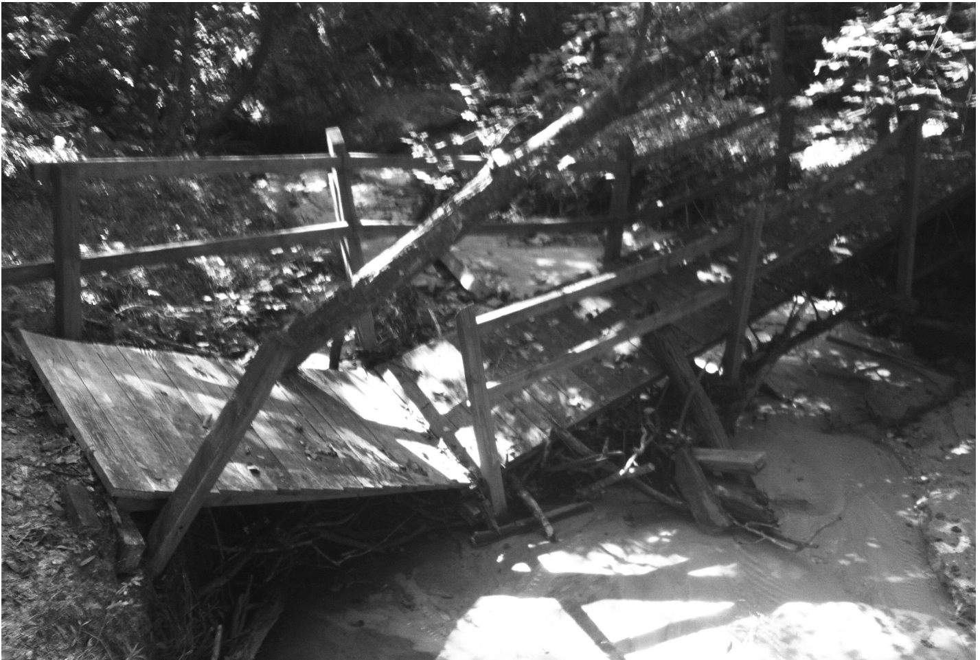
One of the bridges along the Pauline Longest Nature Trail is left in disrepair after a heavy storm.
