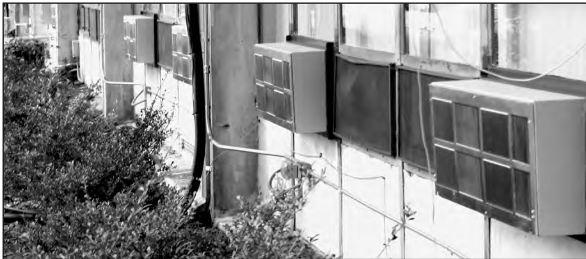
Photo of trustees new air conditioning units by Aaron Bressler
