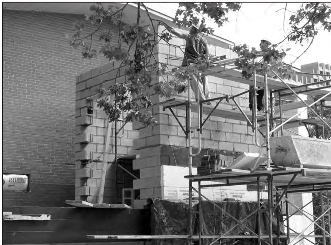
Workers construct the new elevator in the Trustees Building. The elevator is expected to be completed by early November. Photo by Ashley Young.
