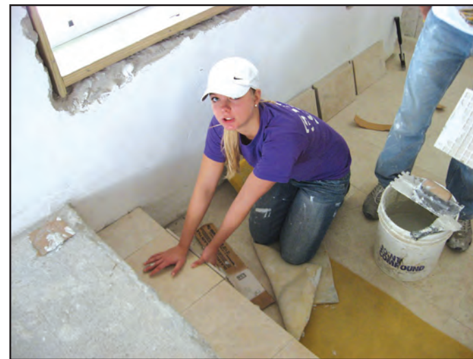
Bottom: Ashley Stoudt pauses while laying tile in a house in the Bahamas. Photo contributed by John Morton.
