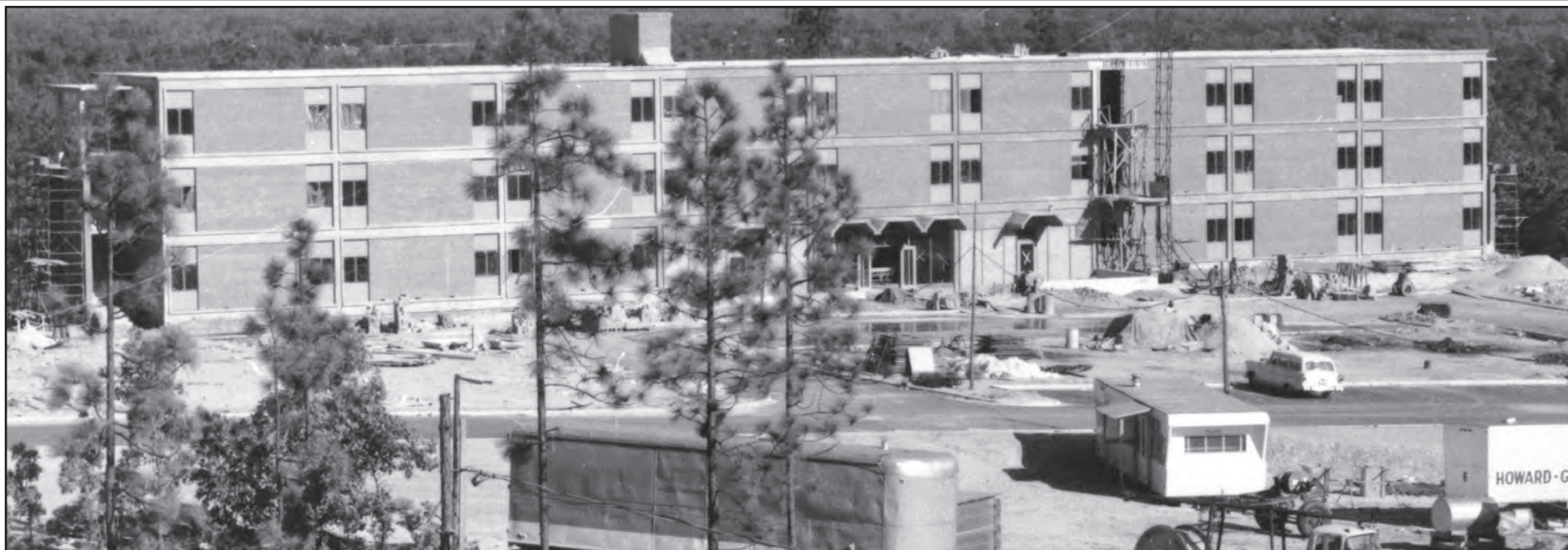
An undated photo courtesy of Bill Billings shows the construction of Cumberland Hall. This hall is considered to be a "traditional hall," which will be restored at the end of the campaign
