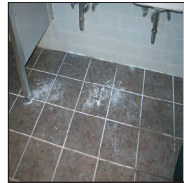
Residue on bathroom floor
